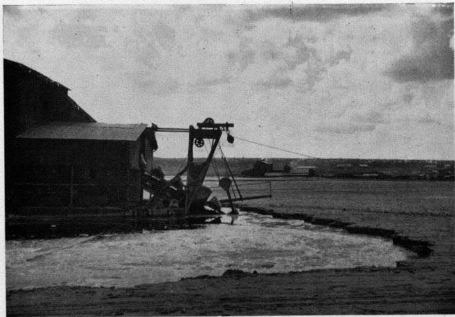
Plate VIb—Dredging trona at Lake Magadi. The trona is pumped to the factory in the middle distance for processing into soda ash
