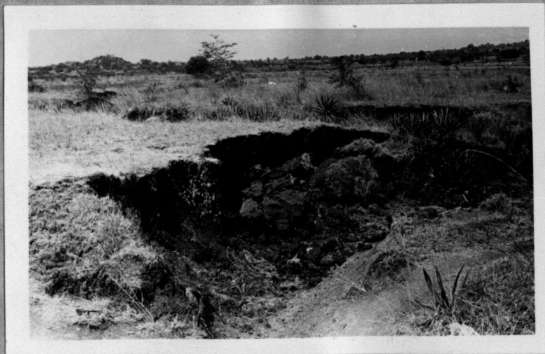
Plate 3. - Erosion gully, in alluvial-lacustrine clays.
