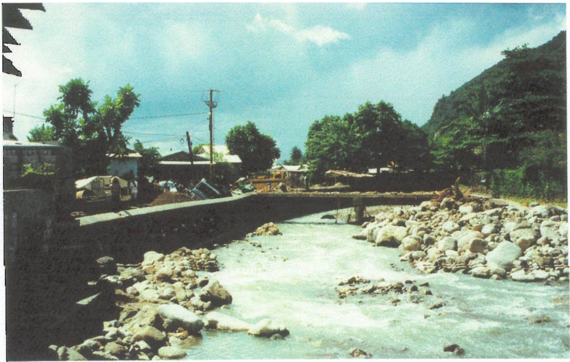
Photo 5 Soufriere Footbridge: Deep girder restricts waterway opening of bridge causing flooding.
