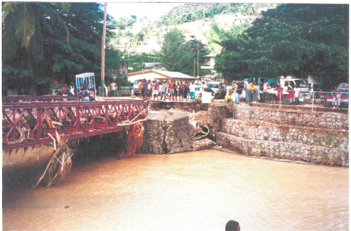
Photo 14 Canaries: Location as per Photo 13 showing abutment collapse after flood of 26th. Oct..
