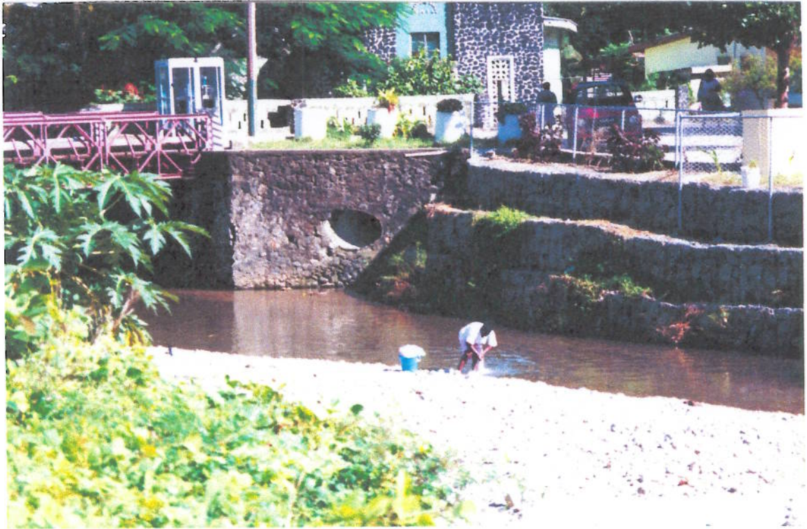
Photo 13 Canaries: Main West Coast Road bridge right abutment before 26th: Poor condition?
