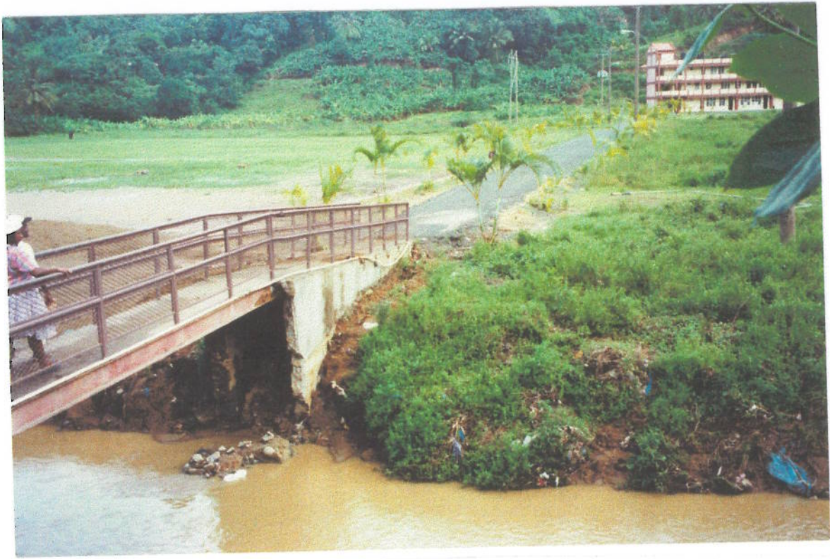
Photo 33 Cul de Sac River : Footbridge access to new Bexon School. Pre October 26th.
