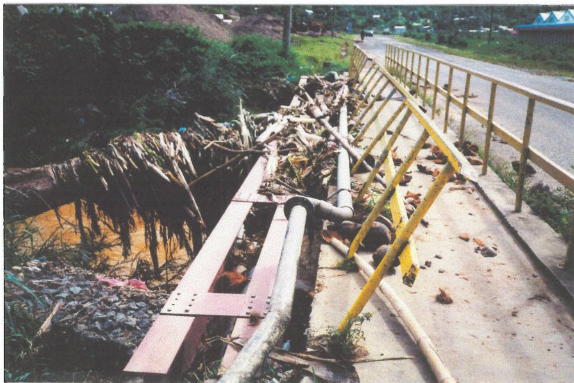
Photo 32 Cul de Sac River. As Photo 31 October 27th. Debris in need of removal. Maintenance?
