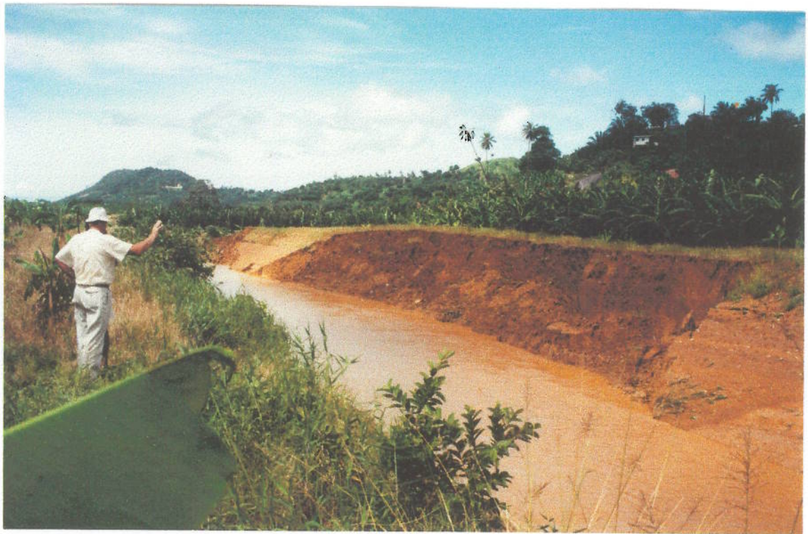
Photo 10 Phase 1 Works: As Photo 9 but after 26th October. Embankment collapse.
