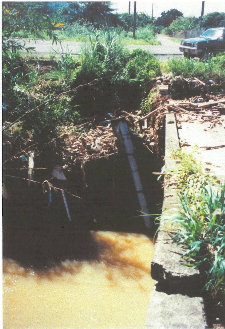
Photo 19 Cul de Sac River. Broken water level recorder station at Ferrands Bridge.
