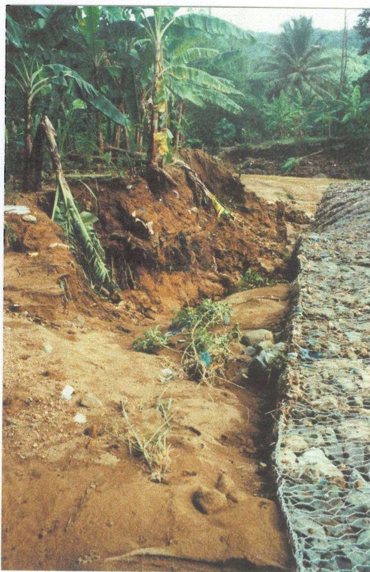
Photo 8 Phase 1 Works: Location as Photo 11- problem of countryside erosion by overtopping.
