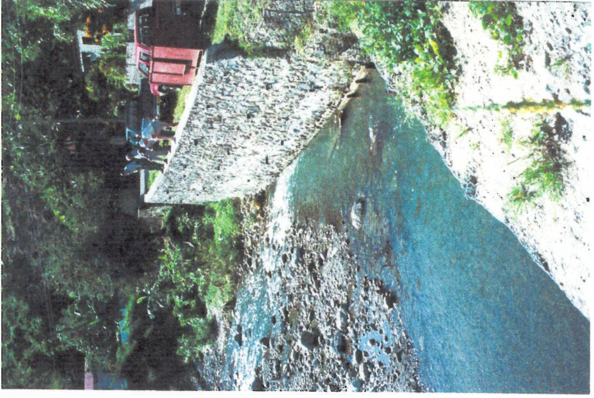
Photo 11 Phase 1 Works: Canaries just upstream of Photo 13. New retaining wall. Gabions fore.
