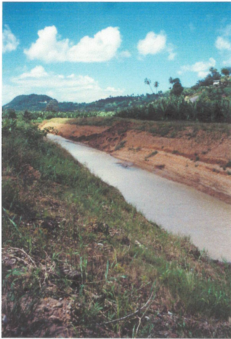
Photo 9 Phase 1 Works: Roseau River south of Belair. Meander loop cut, new straight channel.
