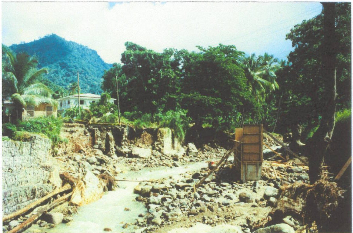
Photo 2 Phase 1 Works: Location as Photo 5. Looking upstream after October 26th flood event.
