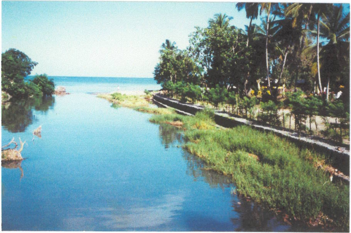
Photo 15 Phase 1 Works: Anse la Raye gabion river training wall ( Glyricidia poles planted).
