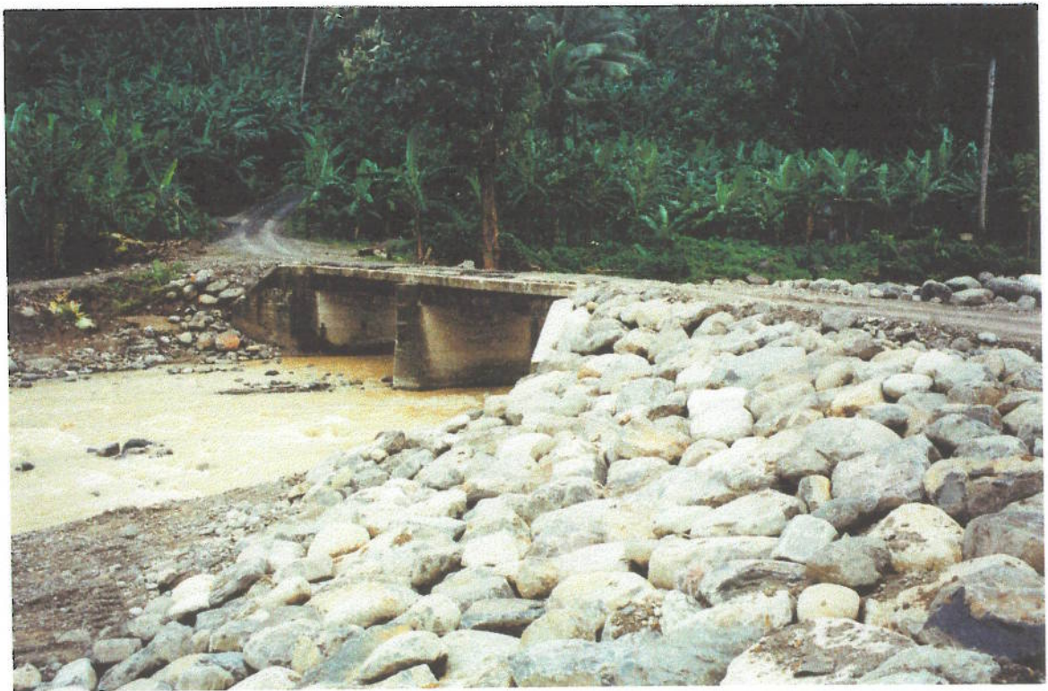
Photo 36 Troumassee River at Mahaut: Novemebr 13th. Bridge reinstated with rip rap protection.
