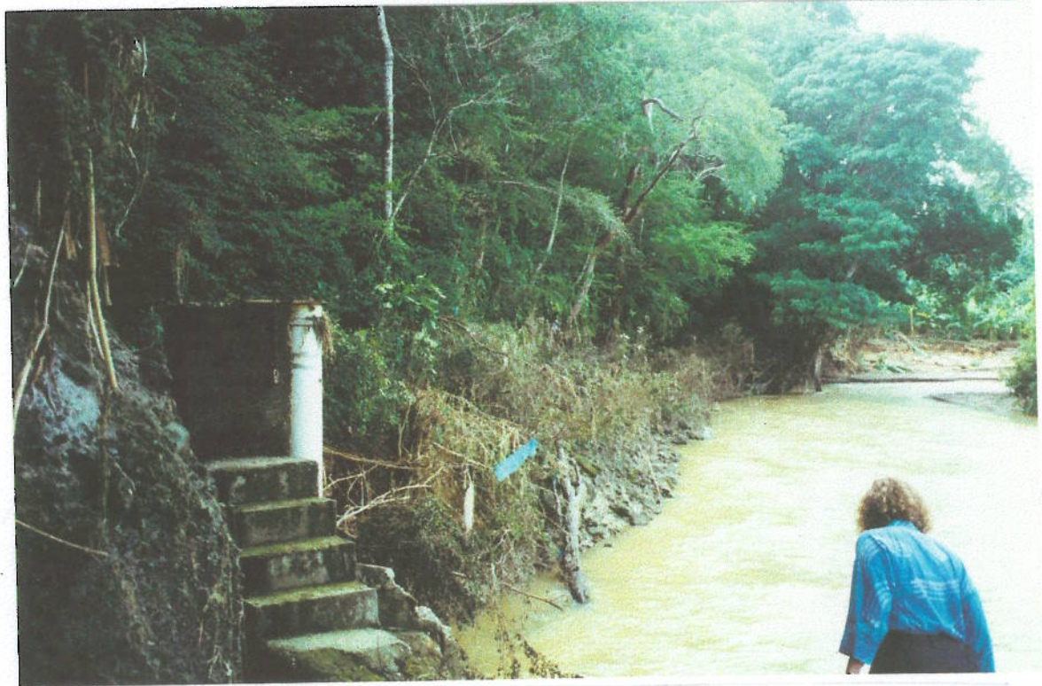
Photo 20 Troumassee River. Broken water level recorder station at Beauchamp Estate.
