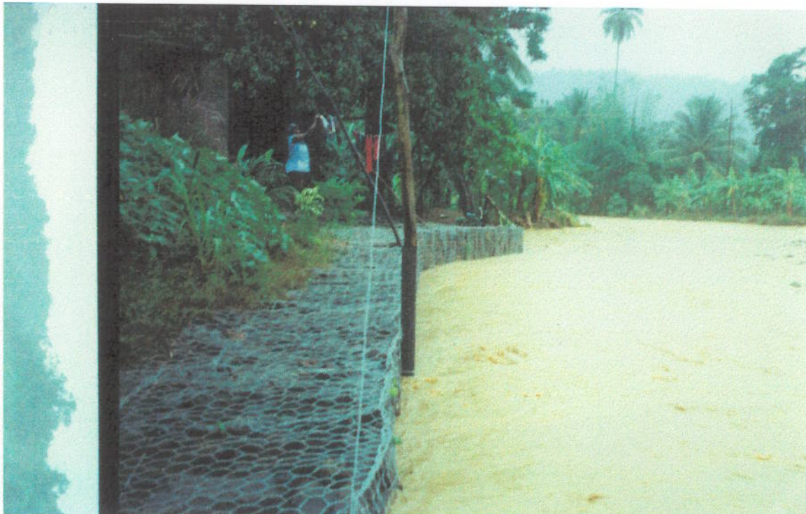
Photo 7 Phase 1 Works: Cul de Sac River near Marc road junction; gabions during event of 26th.
