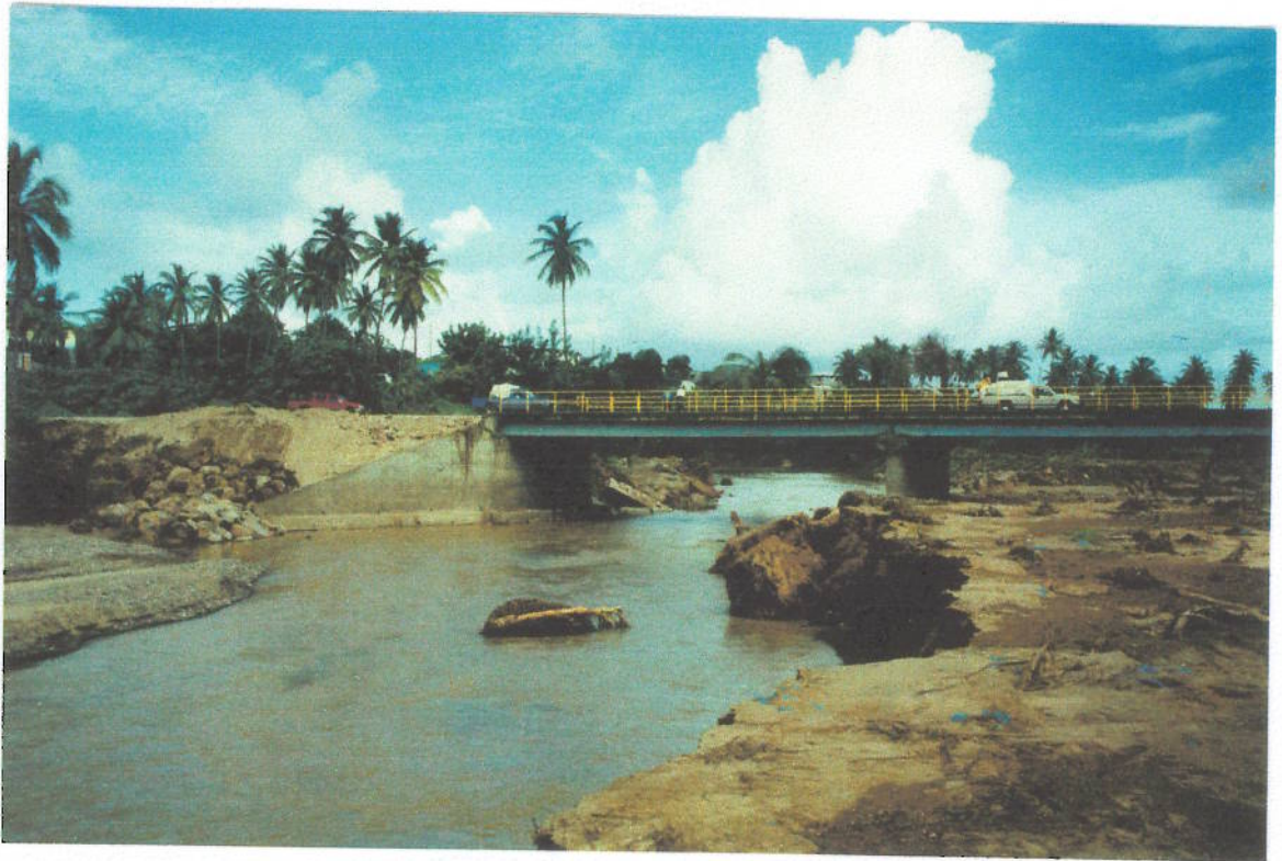
Photo 17 Phase 1 Works: Troumassee Bridge from upstream after October 26th Flood.
