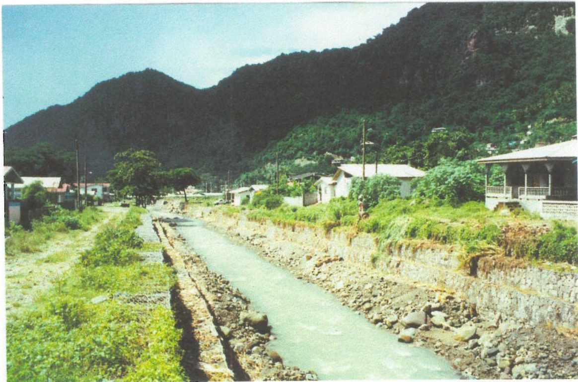
Photo 4 Phase 1 Works: Location as Photo 9 - Flood lowered bed through scour but gabions OK.
